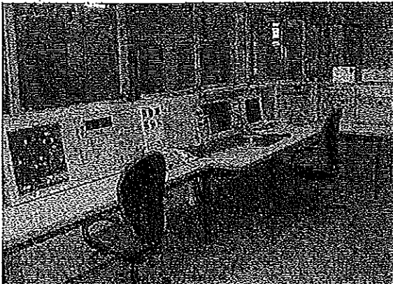
Control station for tests up to 15kA
