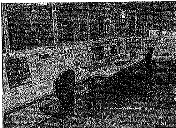
Control station for tests up to 15kA
