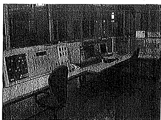
Control station for tests up to 15kA
